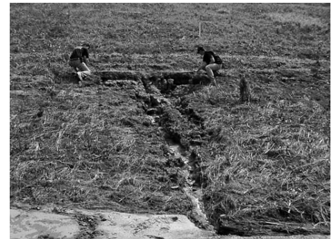
Soil erosion evidence on the downstream face of Florestal Cataguases DAM-B.
